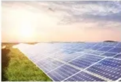
Energy Storage System
