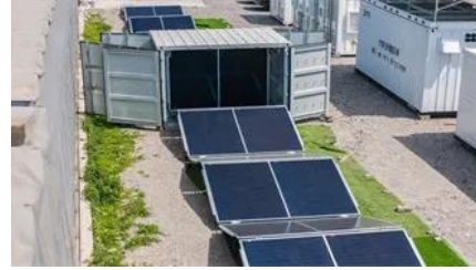
Banjul Lithium Battery Project , PABIANICE BESS
