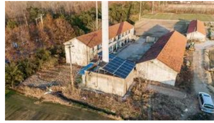
Communication Base Station Wind And Solar Complementary
