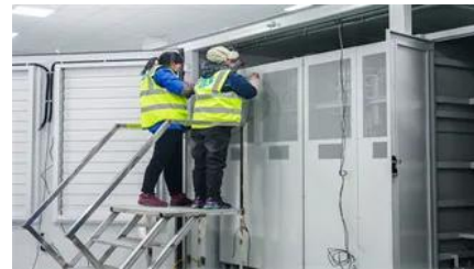
BATTERY ENERGY STORAGE POWER STATION IN BOTSWANA
