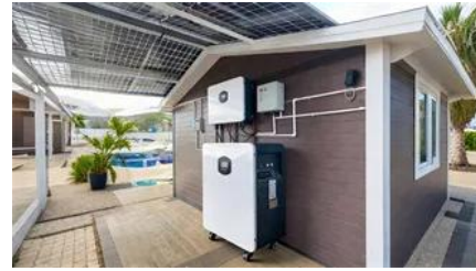
Botswana builds 5G communication base station energy storage system
