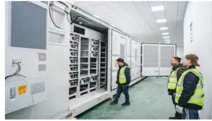
Outdoor Solar System for Bts Telecom Base Station
