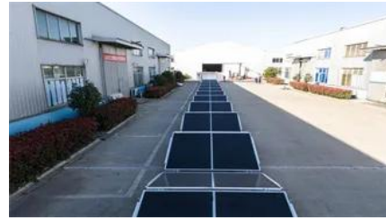
Malta communication base station EMS photovoltaic power generation
