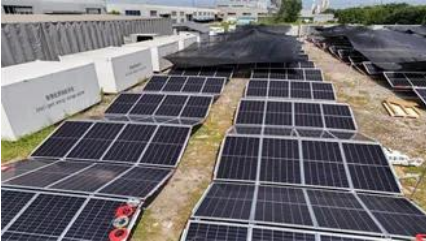
OUTDOOR MODULAR CABINET , Solar Power Solutions
