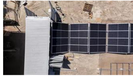
Container Energy Storage Solution / Containerized
