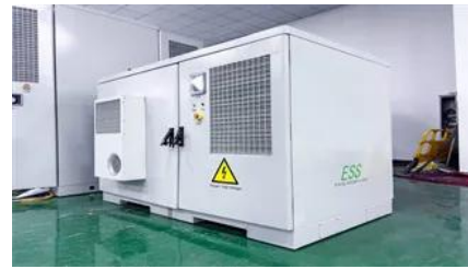
Energy storage container, BESS container
