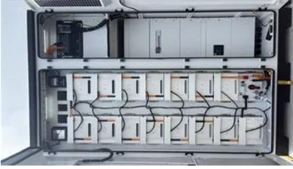
Energy Storage ESS Cabinet with 50kW Lithium
