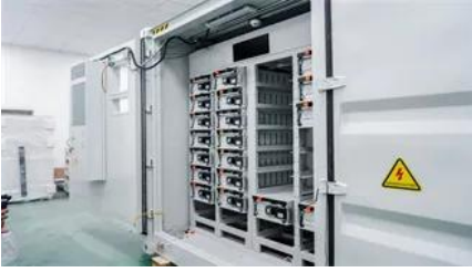
Energy storage container, BESS container
