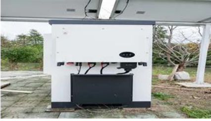
Hong Kong stainless steel photovoltaic bracket power generation
