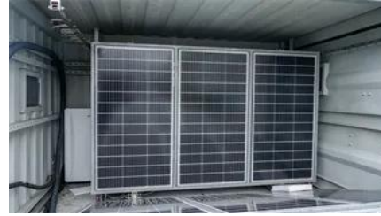
Honiara 2mw Energy Storage Smart Microgrid
