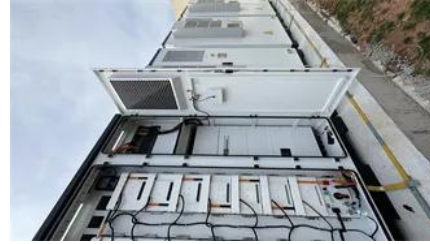
Solar Battery & Inverter Repair Service San Jose, CA , Gecko
