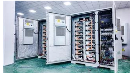
Huawei 48V100AH lithium iron phosphate battery ESM
