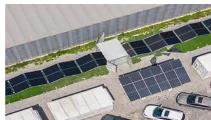
China 113KWH Lithium Battery BESS All In One
