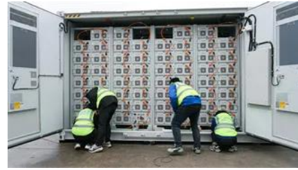
Senegal switches on inaugural solar-plus-storage facility
