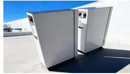
Design and installation of lithium-ion batteries for solar container
