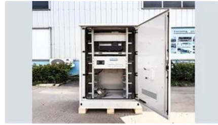
LG Electronics Commercial Energy Storage System 250 kW
