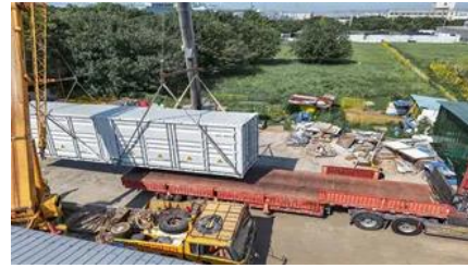
Outdoor Energy Storage Cabinet - solaryyy
