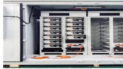
Outdoor Photovoltaic Energy Cabinet, Base Station Energy Storage
