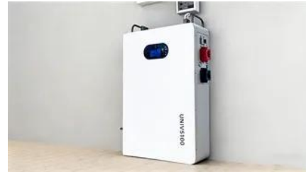
Telecom Base Sites , Hybrid Energy Mobile Wireless Station
