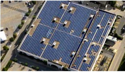
Monocrystalline Silicon Solar Panel , HALKIDIKI BESS
