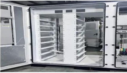
Containerised BESS Energy Storage Solutions , 0.5
