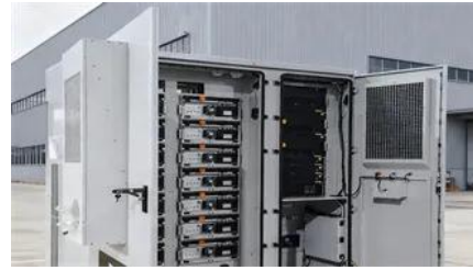
Customized Mobile Solar Container , Portable Solar Energy Storage
