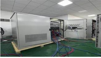
Port moresby energy storage power station tender
