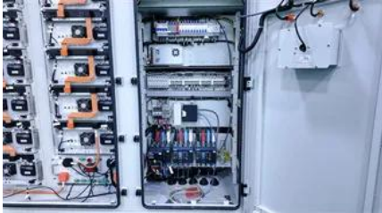
Power devices of port vila energy storage system
