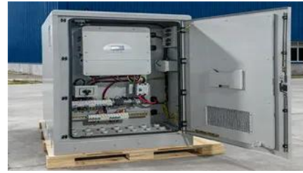
Port Louis Northwest Energy Storage System Integrator: Powering
