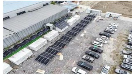
PAPUA NEW GUINEA GRID BATTERY ENERGY STORAGE STATION
