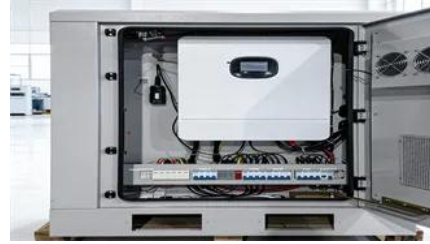
Power supply for Boston Communications solar base station
