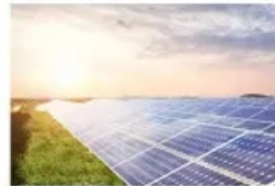
Energy Storage System
