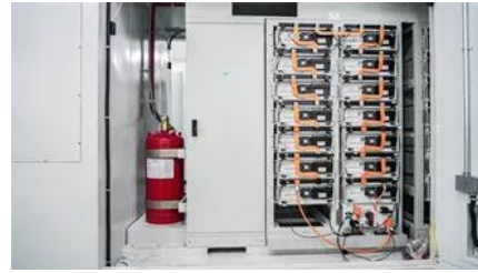
Outdoor cabinets as energy storage enclosure
