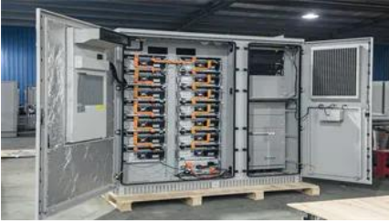
Utility-scale battery energy storage system (BESS)
