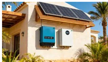
Cambodia 16 kWh Solar Battery Installation: Household
