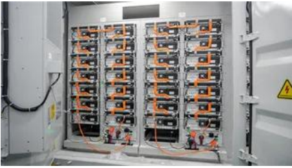
Personal solar container battery structure
