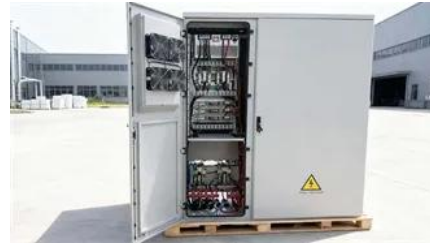
Somalia container communication base station telecom solar site
