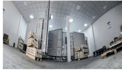
No.1 Capacity Solar Container , Solarabox
