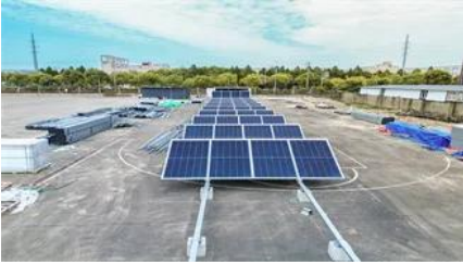
Sudan smart energy storage cabinet center
