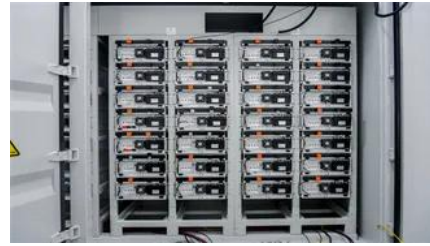
Syria cabinet energy storage system cabinet factory price
