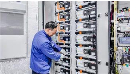
Tirana photovoltaic solar container inverter.
