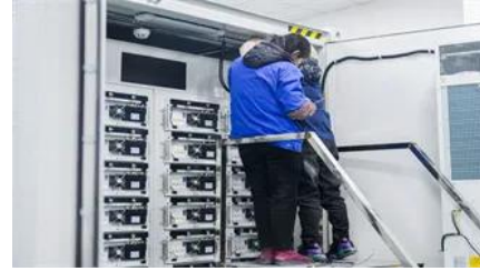
Valletta backup energy storage solar container lithium battery
