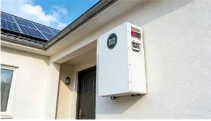
West Africa Steel Battery Energy Storage Container
