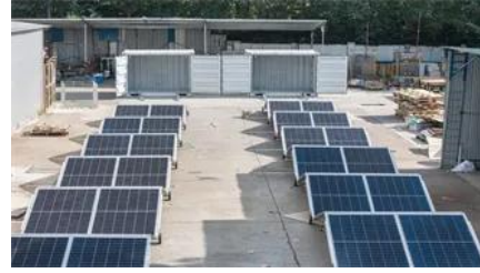
20 FOOT SHIPPING CONTAINERS , WALMER ENERGY
